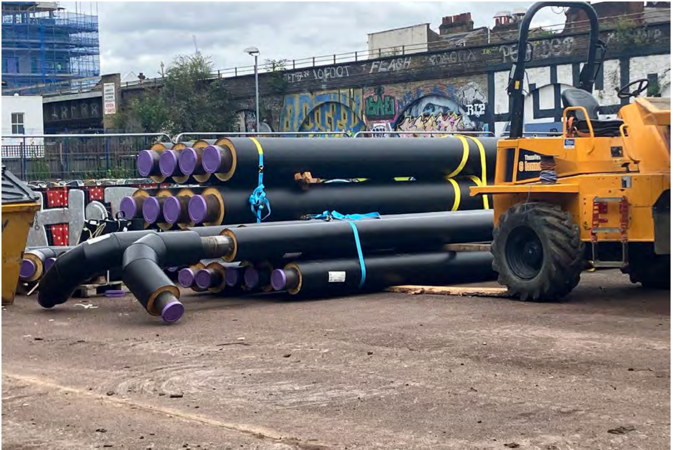
District Heat Network pipes
